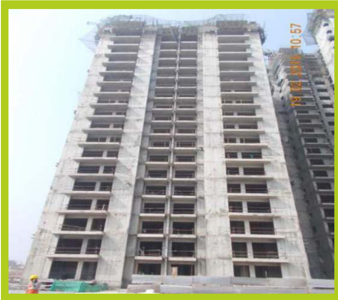
TOWER E February 2015 18th floor slab - 67% completed 19th floor slab - 35% completed 20th floor slab - 35% completed
