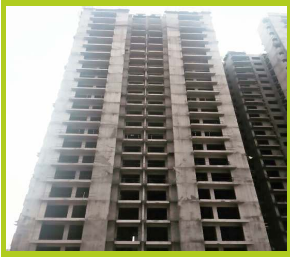
TOWER E June 2015 Super structure completed Interior plaster work under progress Interior finishing work under progress
