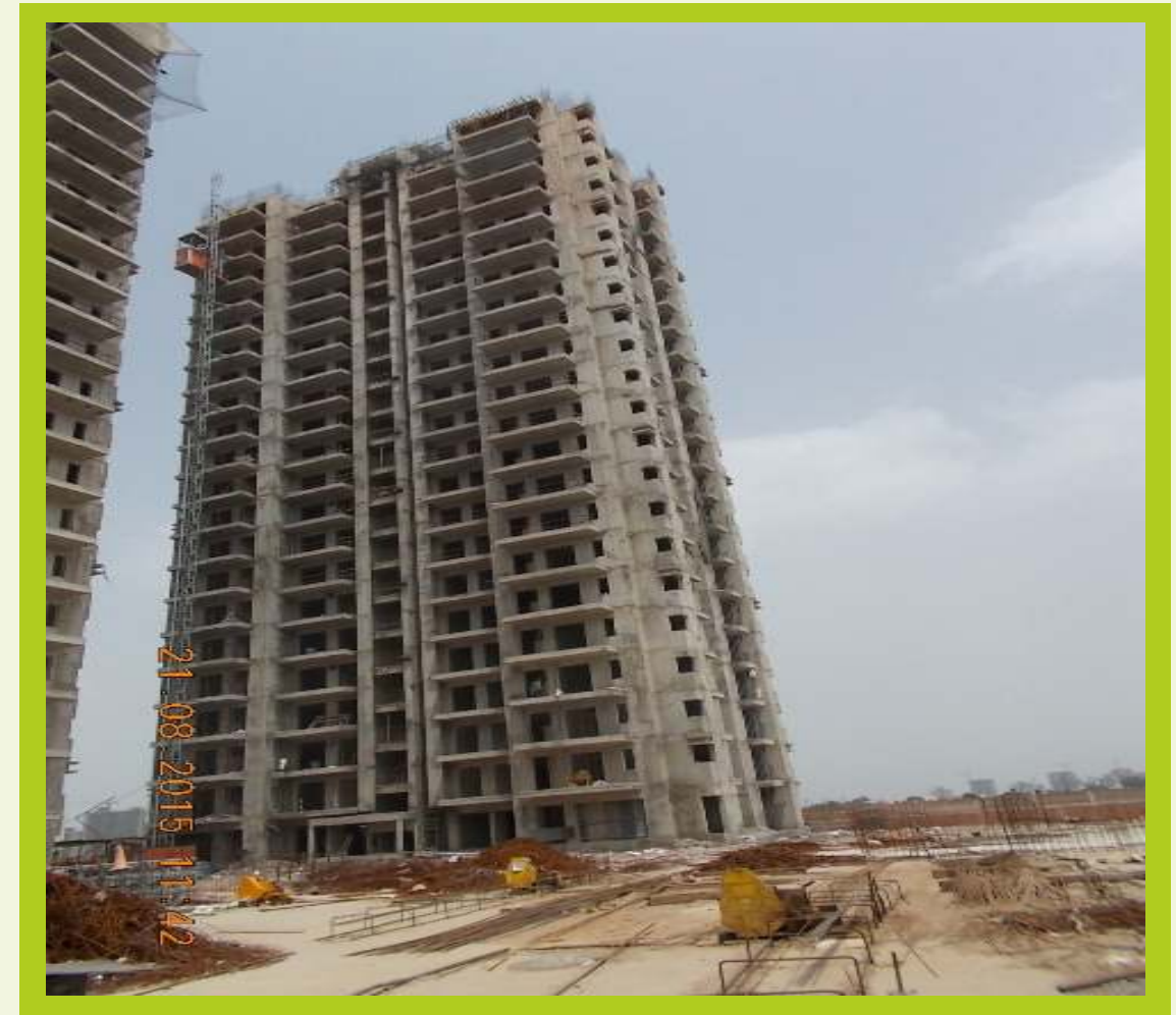
TOWER H August 2015 Super structure completed Interior plaster work completed Interior finishing work under progress
