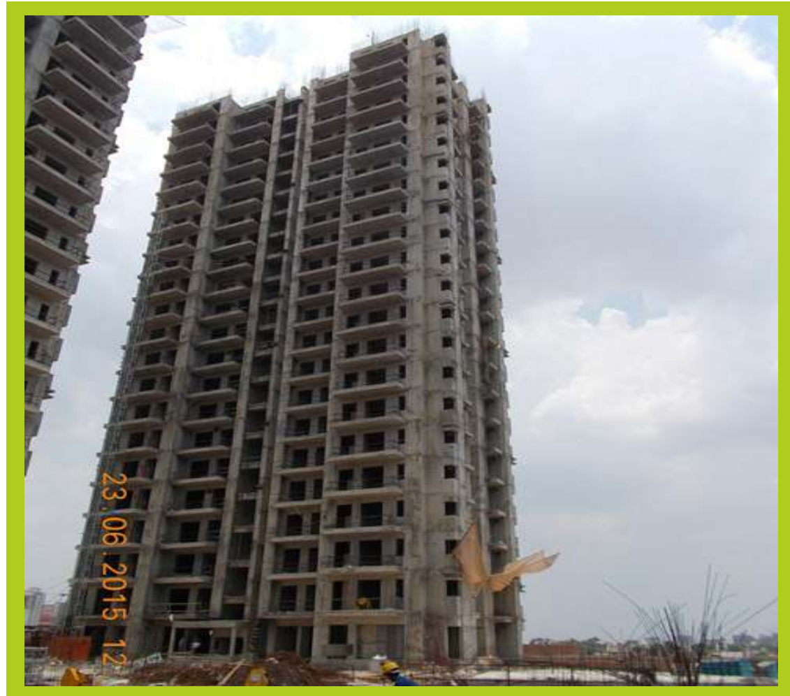
TOWER H June 2015 Super structure completed Interior plaster work under progress Interior finishing work under progress
