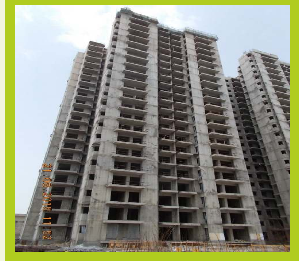
TOWER E August 2015 Super structure completed Interior plaster work completed Interior finishing work under progress
