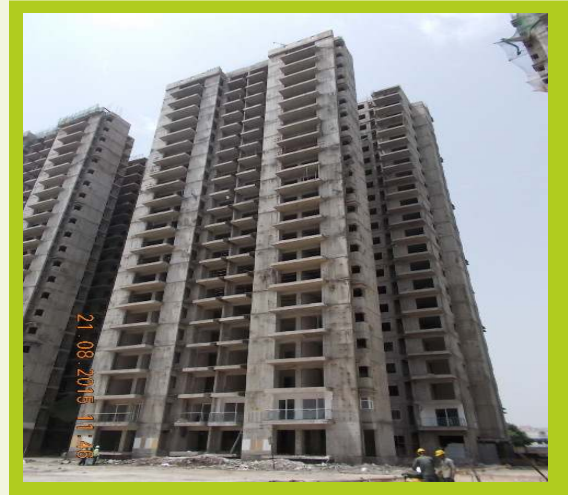
TOWER F August 2015 Super structure completed Interior plaster work completed Interior finishing work under progress
