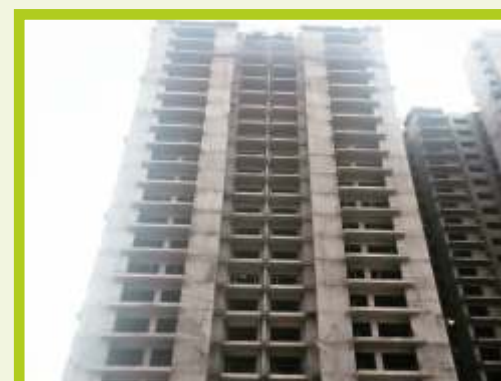
Super structure completed Interior plaster work under progress Interior finishing work under progress
