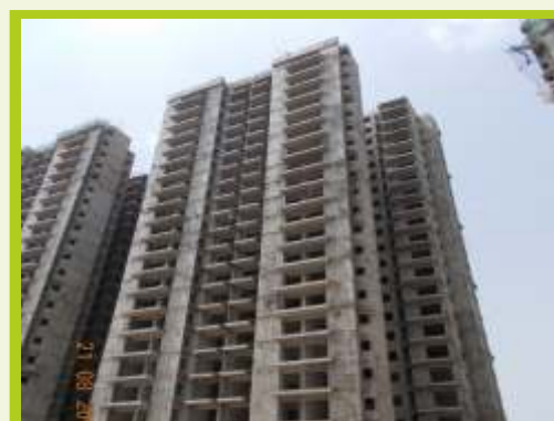
Super structure completed Interior plaster work under progress Interior finishing work under progress
