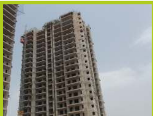
Super structure completed Interior plaster work completed Interior finishing work under progress
