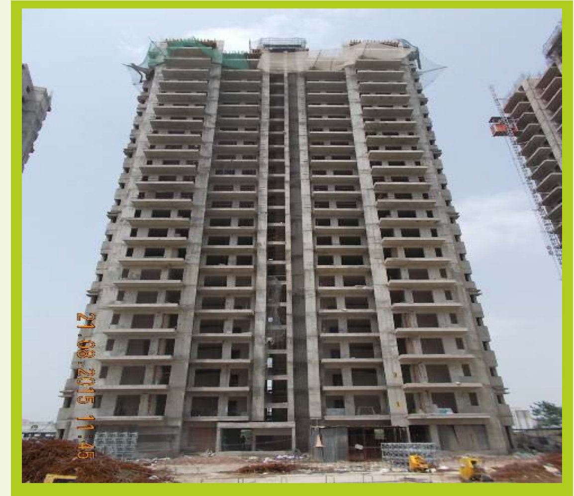
TOWER G August 2015 Super structure completed Interior plaster work completed Interior finishing work under progress
