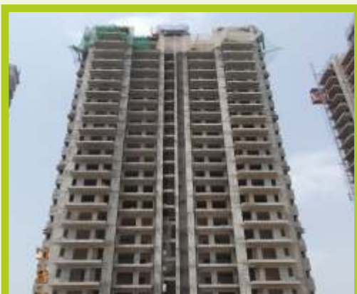
Super structure completed Interior plaster work completed Interior finishing work under progress
